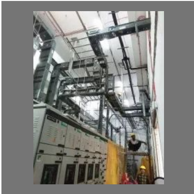
Electrical HT Bus Duct Services
